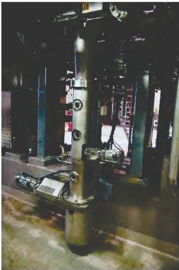
Installation i RTC Pilot Plant
